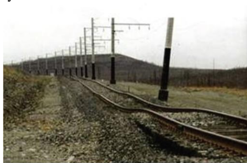
Figure 2. Deformation of the Baikal-Amur Mainline railway.
